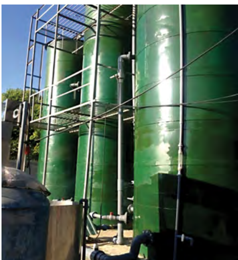
Anaerobic wastewater treatment systems (IC - Internal Circulation)
